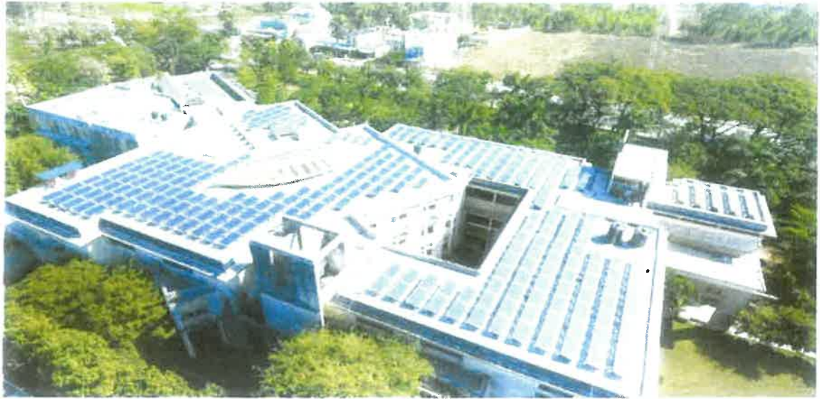
Fig. 9 Photot of Solar Roof Top PV system
