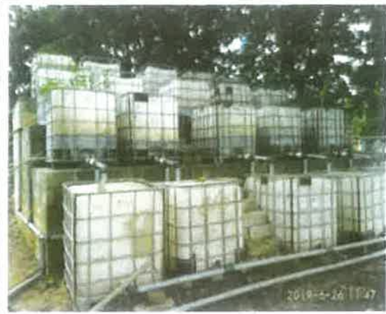
Fig. 5 5kld Phyto-remediation system
