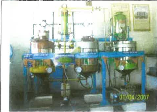
Fig.10 Esterification unit at bio energy center
